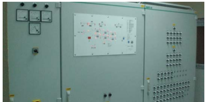
20. MCC-PLC Panel / Pano
