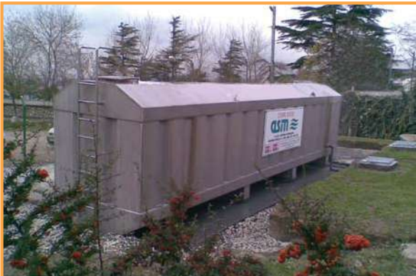
Ambarlı Doğalgaz Çevrim Santrali / İSTANBUL Ambarlı Natural Gas Combined Cycle Plant / İSTANBUL
