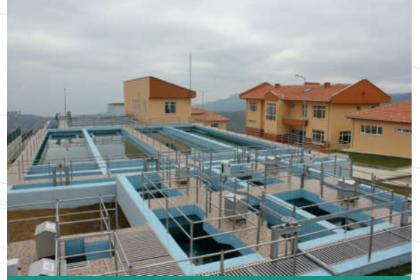
AKÇAKÖY (TRABZON) İÇMESUYU ARITMA TESİSİ AKÇAKÖY (TRABZON) DRINKING WATER TREATMENT PLANT
