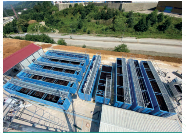
RİZE OSB PAKET ARITMA TESİSİ RİZE ORGANIZED INDUSTRIAL ZONE PACKAGE TREATMENT PLANT
