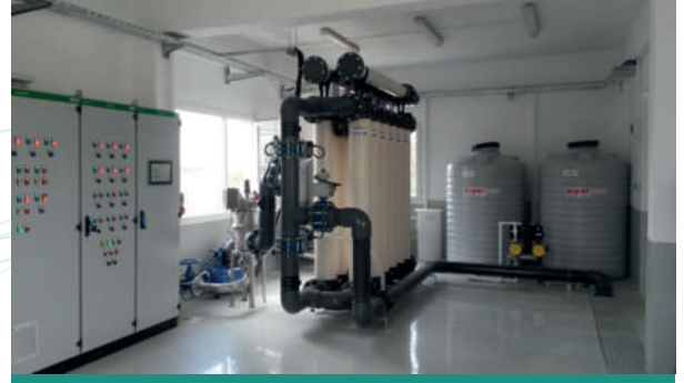
TİRE OSB (İZMİR) ENDÜSTRİYEL ATIKSU ARITMA TESİSİ TIRE ORGANIZED INDUSTRIAL ZONE (İZMİR) INDUSTRIAL WASTEWATER TREATMENT PLANT
