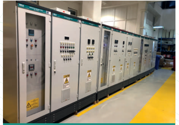
GOBUSTAN (AZERBAIJAN) ATIKSU ARITMA TESİSİ GOBUSTAN (AZERBAIJAN) WASTEWATER TREATMENT PLANT
