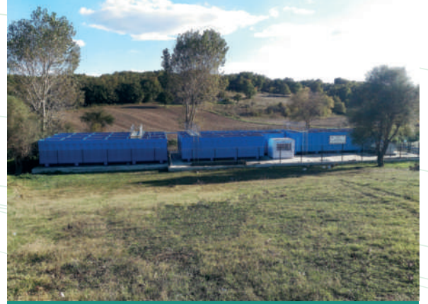
BÜYÜKÇAVUŞLU İSKİ (İSTANBUL) PAKET ARITMA TESİSİ BUYUKCAVUSLU ISKI (ISTANBUL) PACKAGE TREATMENT PLANT
