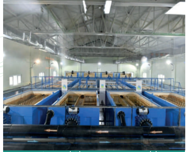
SUSURLUK (BALIKESİR) İÇMESUYU ARITMA TESİSİ SUSURLUK (BALIKESİR) DRINKING WATER TREATMENT PLANT
