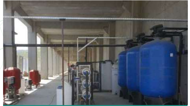
GAMA RECYCLE (DÜZCE) ENDÜSTRİYEL ATIKSU ARITMA TESİSİ GAMA RECYCLE (DÜZCE) INDUSTRIAL WASTEWATER TREATMENT PLANT
